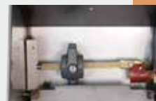
Valve heating (Ref. 131.0527)
