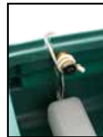
Frost protection heating cable wrapped around the valve
